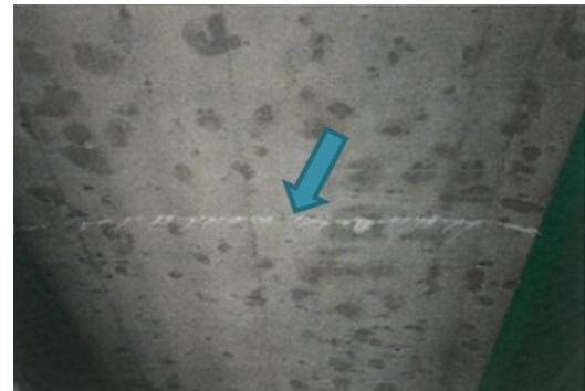
Fig. 1.26 Efflorescence in penetrating transverse cracks (Photo Courtesy: Yokogawa Bridge Holdings Corp.)
