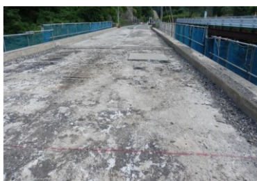
Fig. 1.4 RC bridge deck deteriorated (Exposed rebar and aggregation) due to the action of ASR[5]
