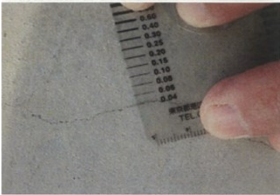
Top Surface Crack 18
