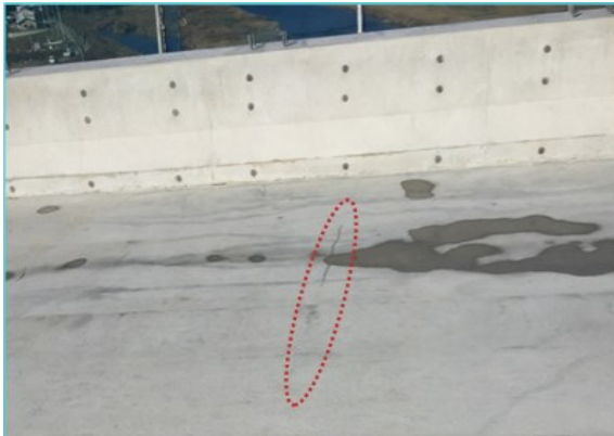
Fig.4.6(a) Minor transverse cracks observed after removal of curing sheet in Lot 2
