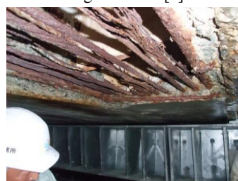
Fig. 1.8 Large amount of deicing salt accelerates rebar corrosion in bridge RC slabs[5]
