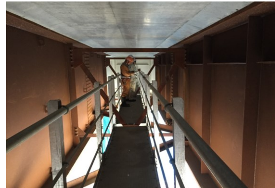
Fig. 1.10 Structural restraints due to undereath steel girdes (Mukai-Sadanai bridge, Kamaishi)
