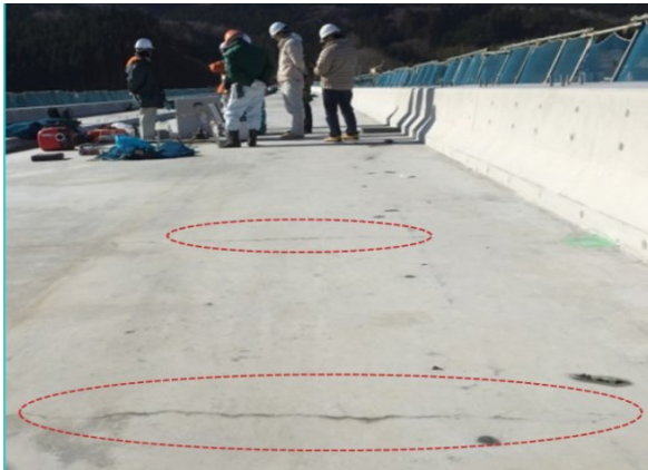
Fig.4.5(a) Minor transverse cracks observed after removal of curing sheet in Lot 1
