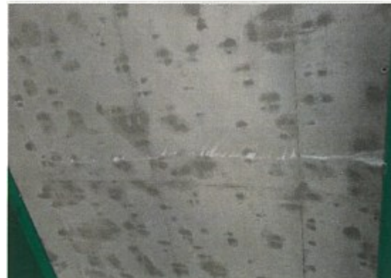
Fig.4.5(d) Bottom surface crack in Lot 1 (Crack 22) showing efflorescence[4]
