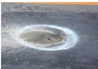
Fig. 1.3 Damages in RC deck slab due to fatigue caused by repeated loading (traffic=12000 vehicles/day)[4]
