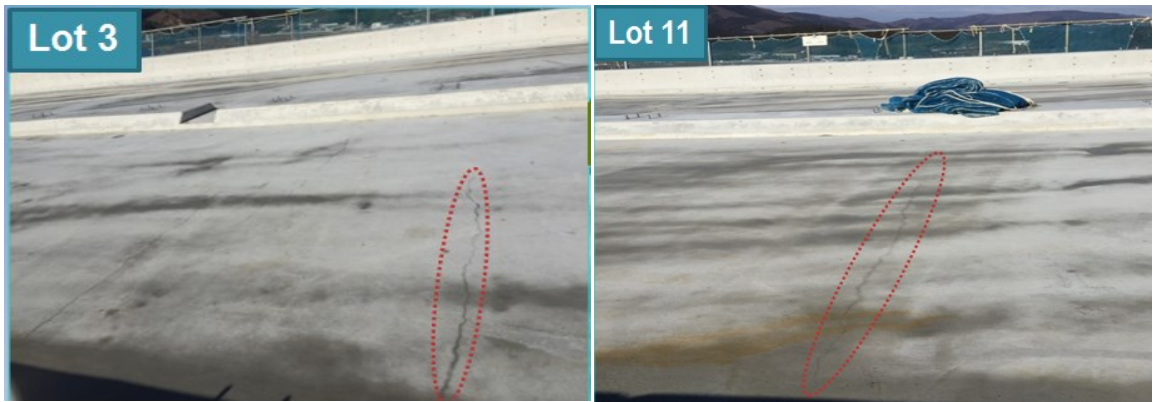
Fig.4.7(a) Minor transverse cracks observed after removal of curing sheet in Lot 3
