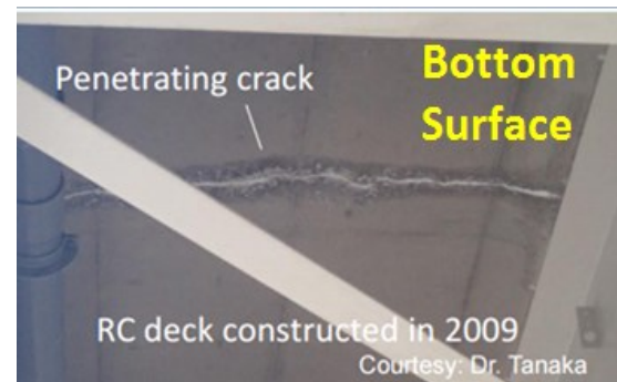
Fig. 1.12 Efflorescence along the penetrating transverse crack in RC slab[5]
