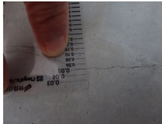
Fig.4.5(b) Top surface crack width measured in Lot 1 (Crack 39)[4]
