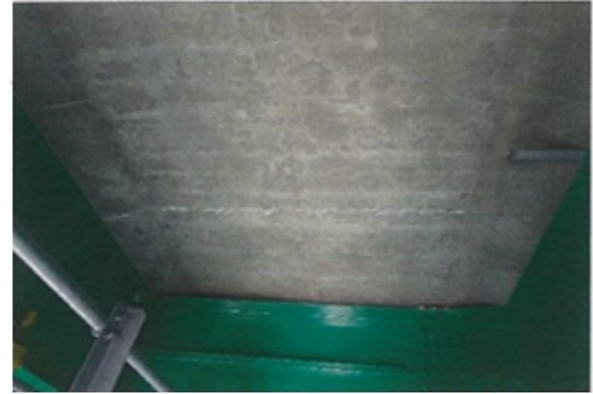
Bottom Surface Efflorescence Crack 4
