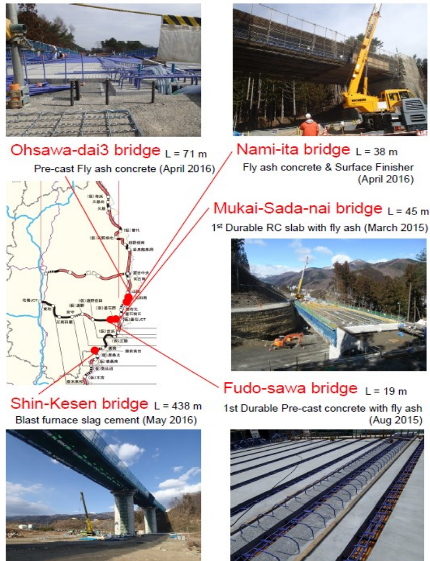
Fig. 1.20 Several durable RC slabs on bridges along Revival Roads adopting multiple protections concrete design [2]
