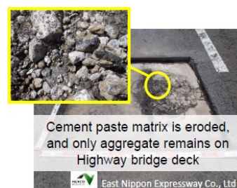
Fig. 1.5 Combined deterioration due to ASR, de-icing salt, repeated load, water migration etc. [5]
