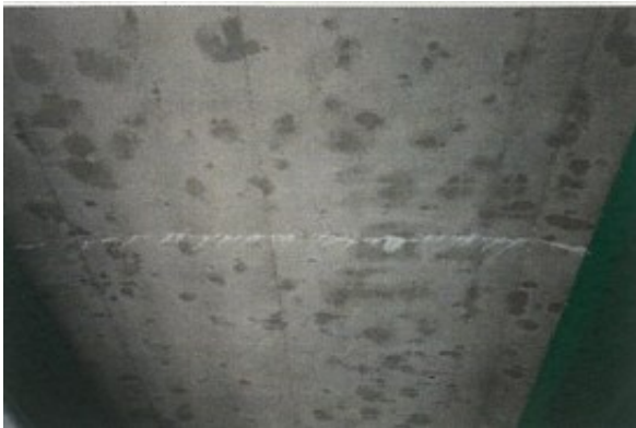
Fig.4.5(c) Bottom surface crack in Lot 1 (Crack 5) showing efflorescence[4]
