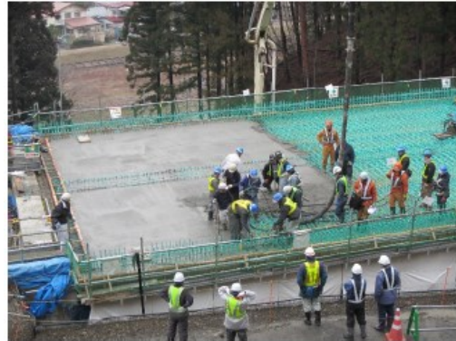
Fig. 1.17 Concrete casting at single span Mukai-sada-nai Bridge (Length=43.7m constructed in March 2015) (First trial contraction of durable RC slab) [2]
