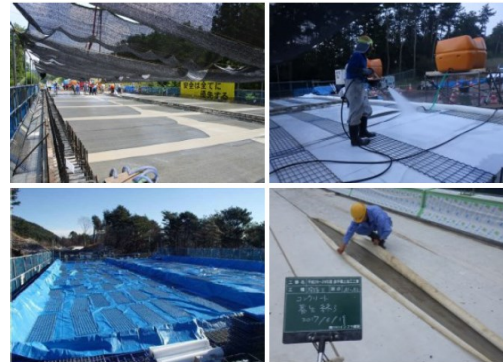
Fig. 1.18 Application of multiple protection concrete design in RC slab construction of single span Hikohei Bridge in Fukushima (Length=43.7m concrete placement in July,2017) [7]
