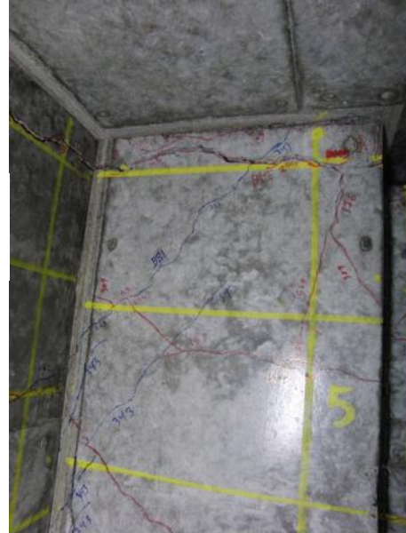
Fig (5.22) Widening of cracks from loading cycle of 1/50 rad
