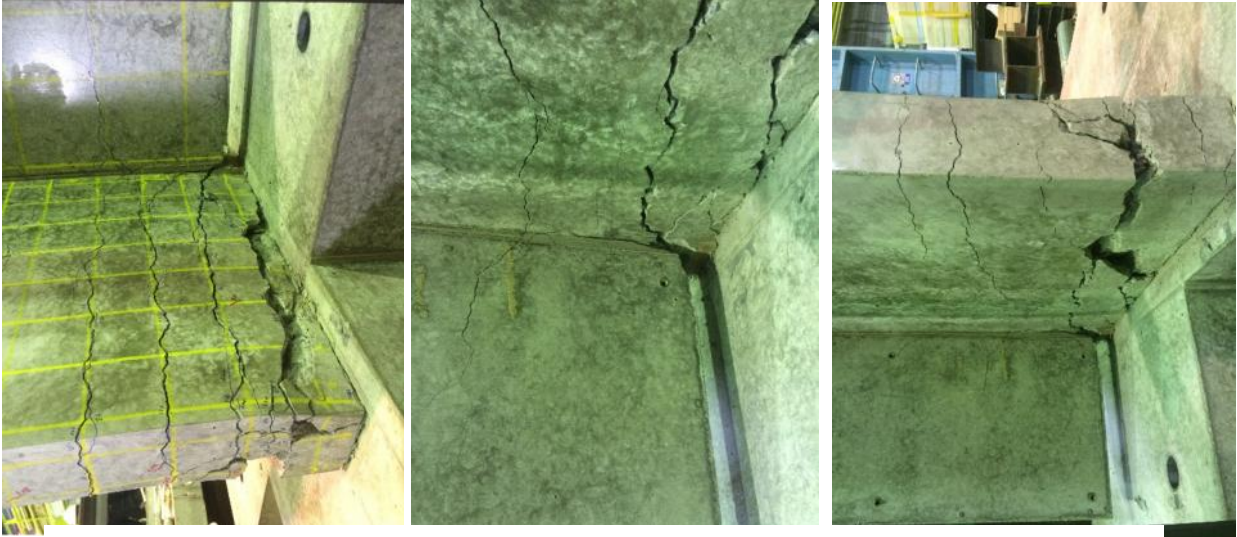
Fig (5.17) Wide cracks with crushing of concrete in the slab
