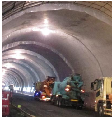
Figure 3.9 Installation of plastic sheet to prevent friction between construction joints between blocks
