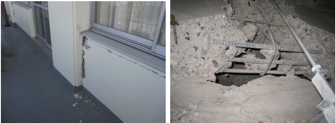
Figure 1-6 Damage in beams [1-9]
