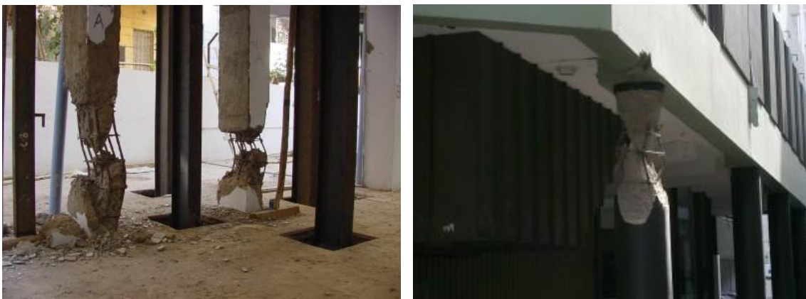
Figure 1-12 Non-ductile RC column failure
