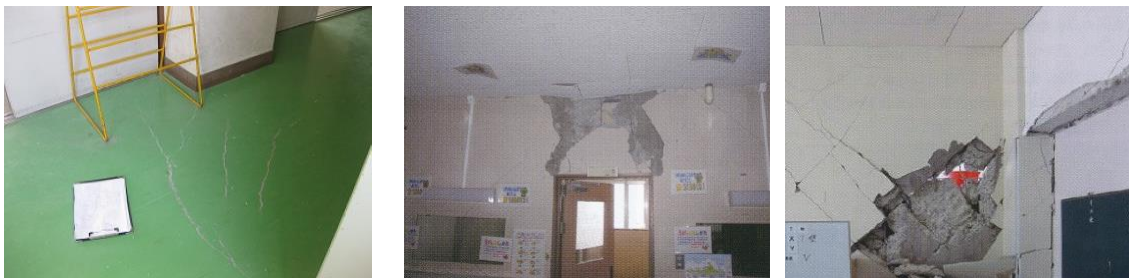
Figure 1-3 Common damage in Structural walls and slaps [1-9]
