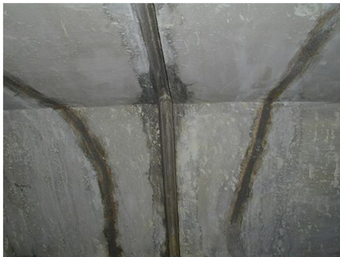
Fig. 1.1 Severe thermal cracks in concrete with slag cement type B and limestone.
