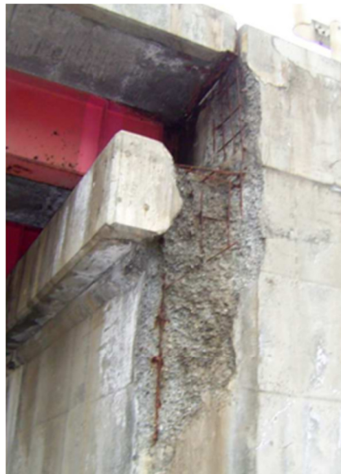
Fig. 1.2 Severe reinforcing bars corrosion.
