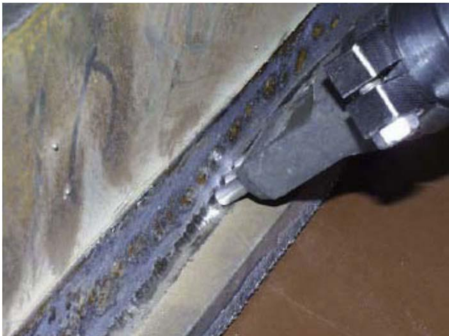
Figure 2.7 Ultrasonic impact treatment of a weld toe in progress (Lihavainen et al. [28]).
