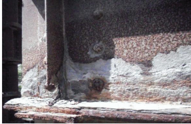
Figure 5.1: Bearing stiffener damage due to corrosion
