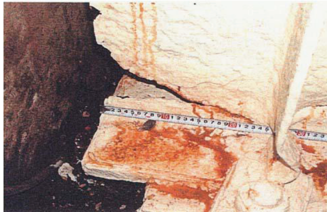
Figure 5.2: Buckling of bearing stiffener caused by section loss (Murakoshi, 2006)
