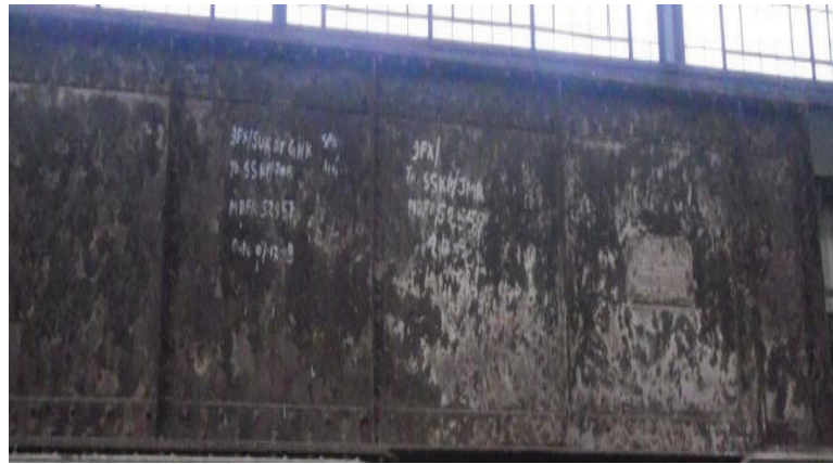
Figure 3.7: Uniform corrosion on steel bridges near sea line areas
