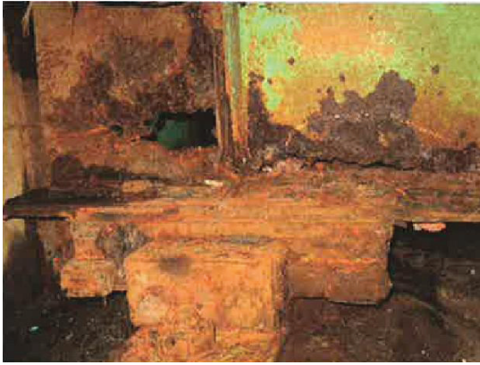
(a) Damage case in Japan (Tamakoshi 2006a)
