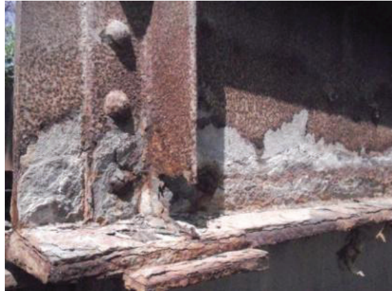
Figure 6.2: Complete loss of bearing stiffener by Khurram (2012)
