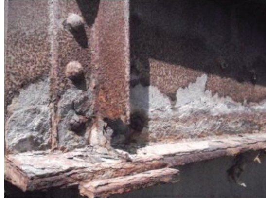
(b) Damage case in Pakistan
