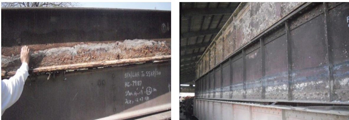
Figure 3.8: Uniform corrosion on the lower portion of web and bottom flanges
