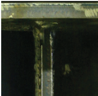
(a) Uniform damage
