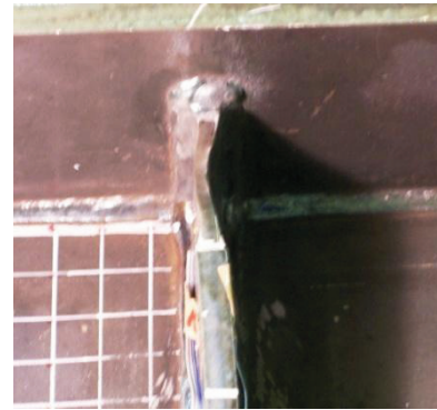
Buckling in Stiffener
