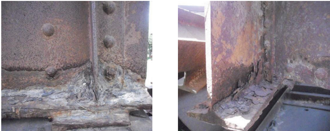
Figure 3.10: Damages at plate girder end due to deposited corrosion
