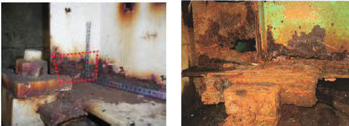
Figure 6.1: Typical corrosion damages at plate girder end by Tamakoshi (2006b)
