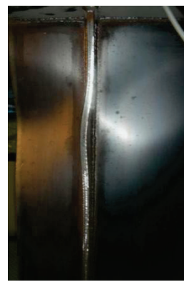
Buckling in Stiffener
