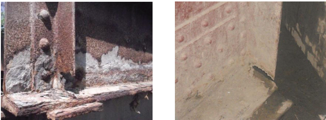
Figure 3.9: Damages at plate girder end due to rain and drainage water accumulation
