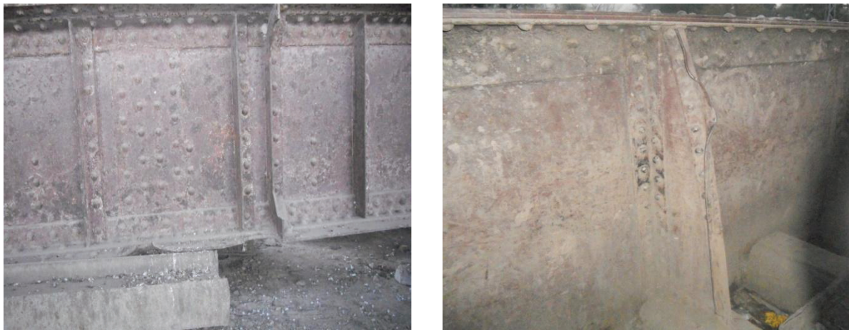
Figure 3.4: The corrosion on the girder due to non-painting
