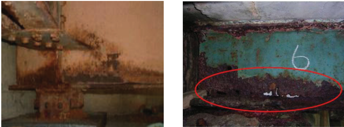
Figure 2.7: Actual corrosion damage cases on plate girder end (Tamakoshi 2006b)
