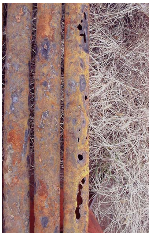
Fig.1-8 Corrosion of 13%Cr SS tubings
