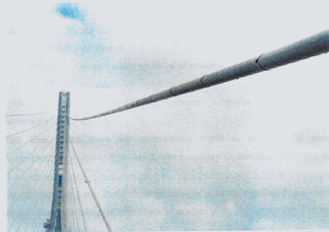
Photo.1.2 Coverings made of colored polyethylene pipe
