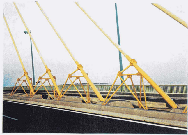
Photo.6.1 Oil-damper of the Brotonne Bridge
