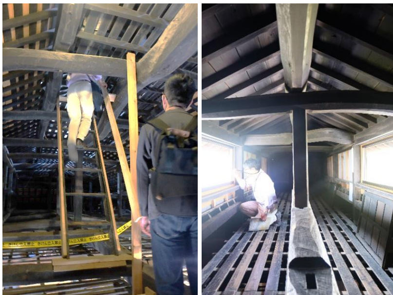
Figure 3-11: Sceneries in a yagura . (Left) A visitor climbing into the yagura of Tajima Zen-ichi Residence omoya . (Right) Space inside a yagura . (Taken by author on May 19, 2019)
