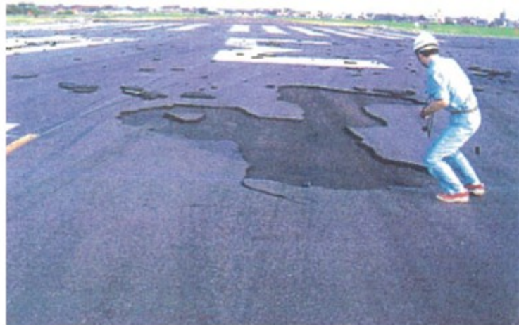
Figure 1.3 Stripping of pavement surface an airport runway
