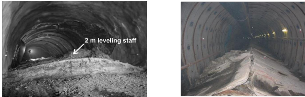
Figure 1-1 Invert heave damage caused by swelling of expansive strata under the tunnel (Butscher et al., 2011)
