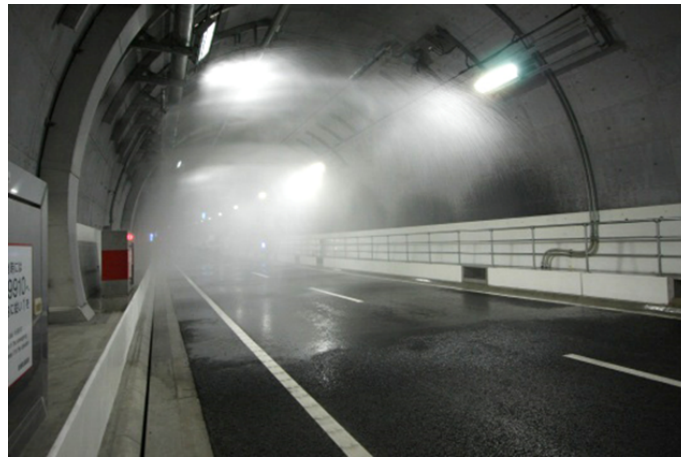
Figure 5.12: Mist operation in tunnel
