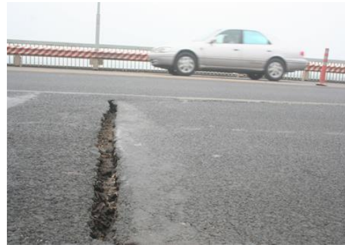
(b) Transverse crack
