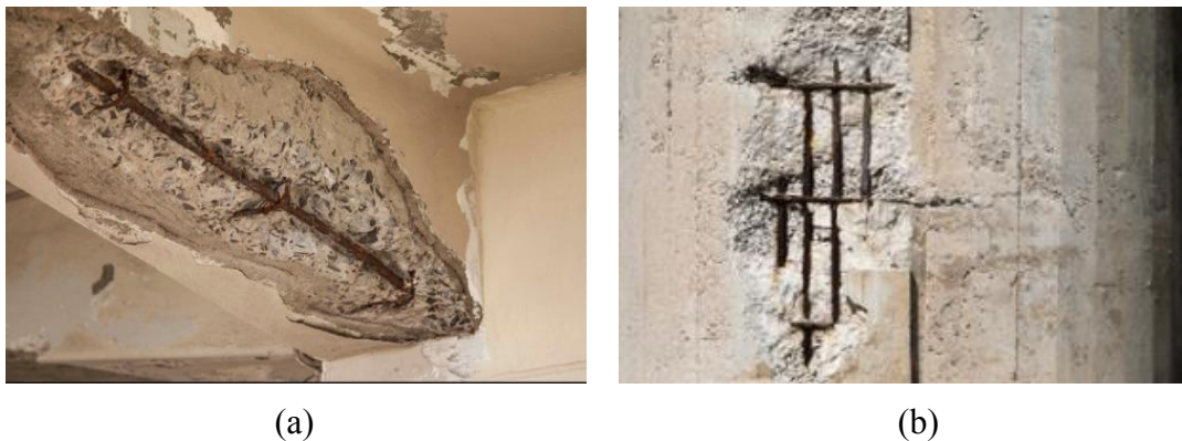
Fig.1.1 Durability problems: (a) Spalling of covercrete; (b) Corrosion of Reinforcement [1.1]
